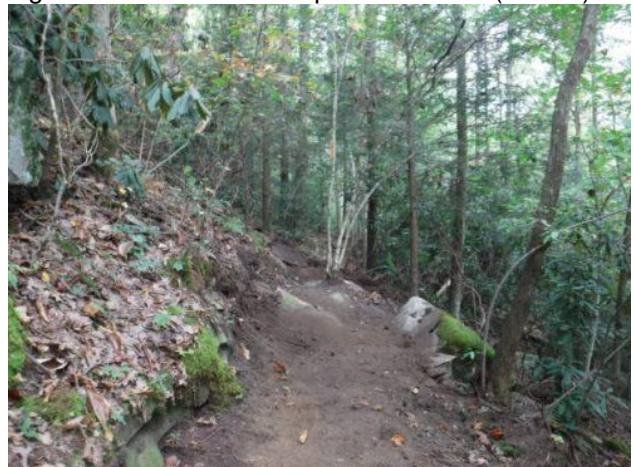
Finished trail on 42 percent side slope above Fall Creek. Ozone Section nears completion October 2019. (Wilson)
